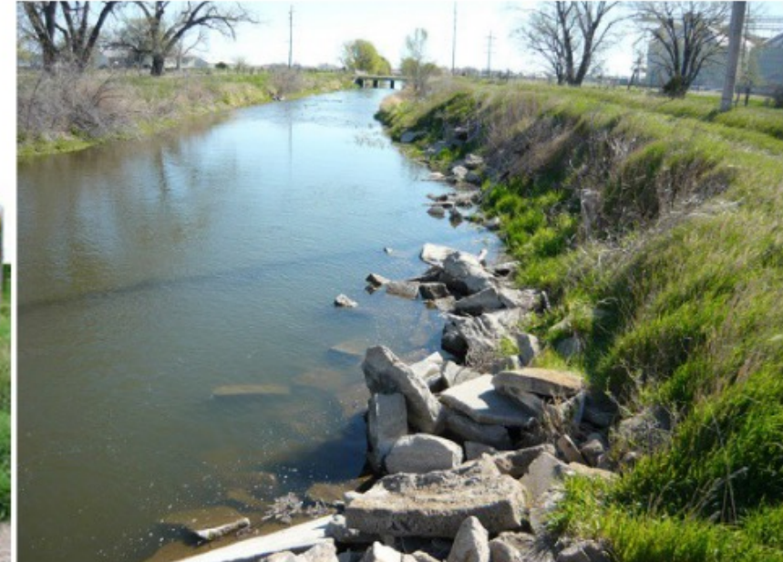
(2014): Channel at headworks holding water as designed.
