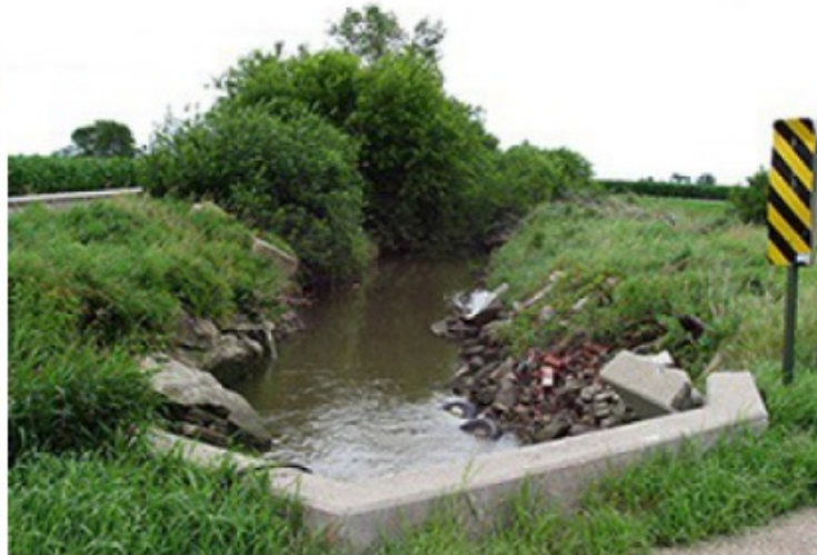
(2012): Channel overgrown with trees and channel in disrepair.
