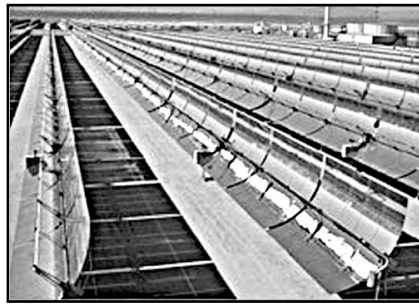
Parabolic trough power plants use a large field of parabolic trough collectors that track the sun and concentrate the solar radiation on a receiver tube located at the focus of the parabolic shaped mirrors.
