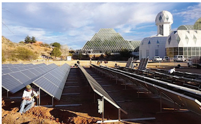
Biosphere 2 solar array project site. Photo credit: Biosphere 2.
