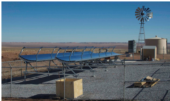
Pilot solar desalination installation on the Navajo Nation. Photo credit: Ardeth Barnhart.
